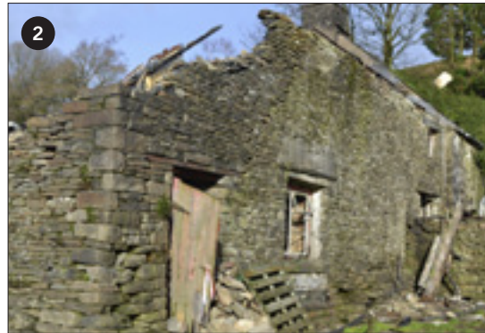
1 Winstanley Hall, Lancs where the Society sought a solution to the building's future.
