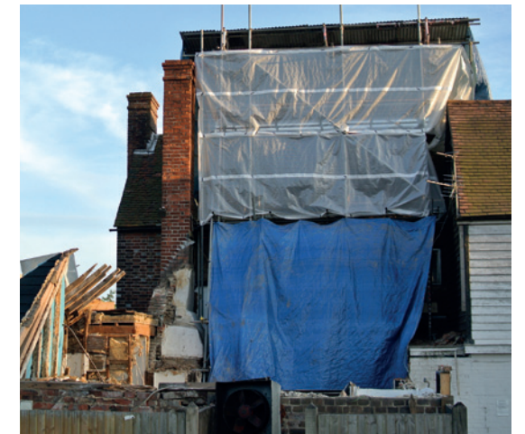
Blue Boys Cafe, Matfield, Kent was partially demolished while under consideration for listing (Iain Boyd/SPAB)
