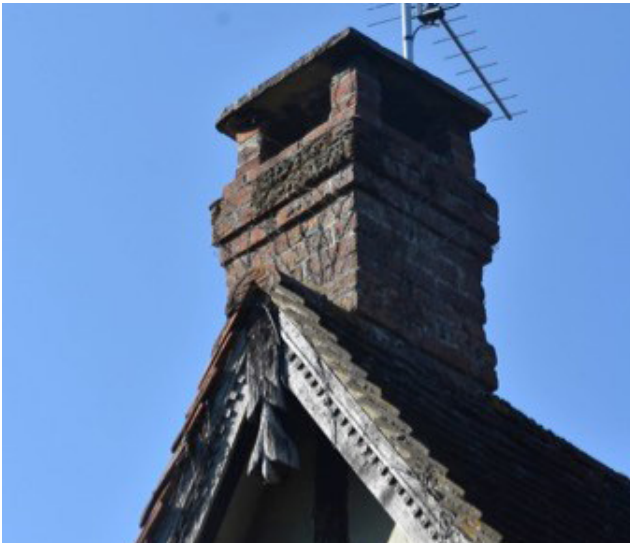
Figure 21: A 'dovecote' top can be used to protect large flue outlets from wind and rain, though is inadvisable on thatched buildings. A stone slab is placed above the flue opening raised on bricks at the corners. Such terminations should incorporate suitable bird mesh to stop nests being built under the slab. However, addition of a slab roof may affect the draw in certain situations. Always light a fire and check for unintended consequences before striking the scaffolding around the stack.
