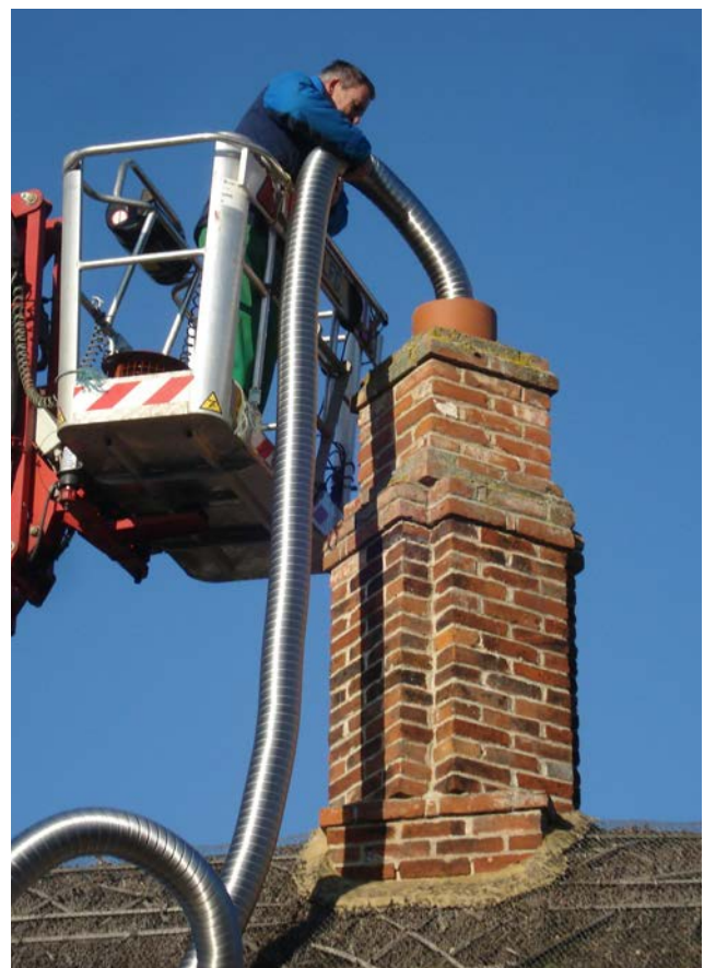
Figure 29: Flexible metal liner being inserted into chimney of thatched cottage to serve new gas stove after removal of a wood burner to reduce the fire risk.
