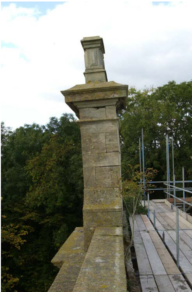
Figure 33: Structural instability. Photo: © Douglas D Kent
