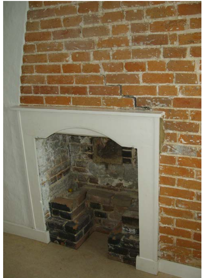
Figure 24: Cracking to chimney brickwork. Photo: © Douglas D Kent
