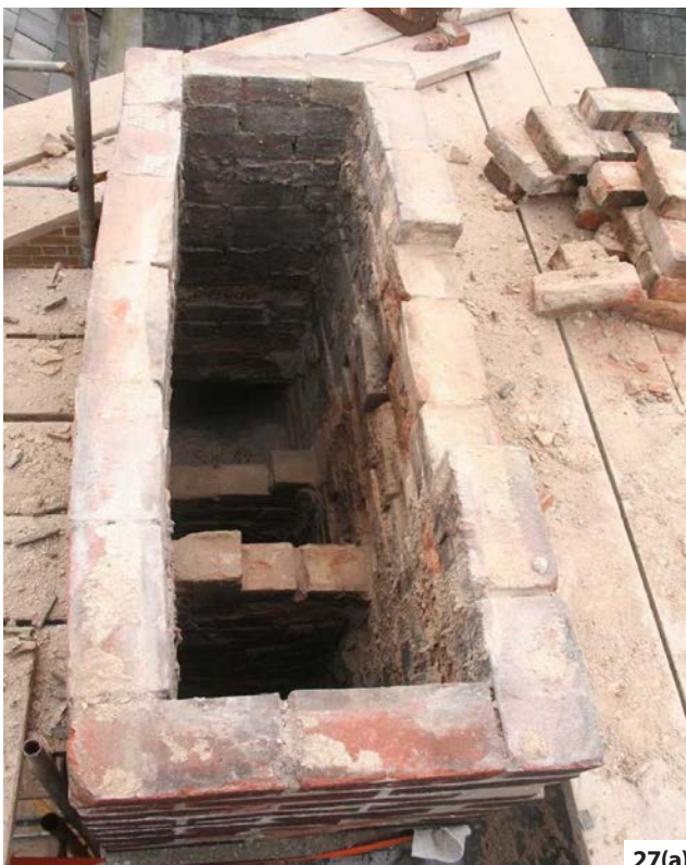
Figure 27: Withes: (a) Part-dismantled during repair. (b) After repair.
