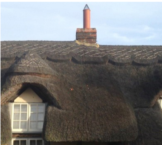
Figure 32: A chimney terminating less than the recommended 1.8 m above the ridge of a thatched building. The top of the terminal with an uninsulated pot is taken as being 150 mm above its base. The addition of a bird guard will reduce fire risk. Photo: Marianne Sühr
