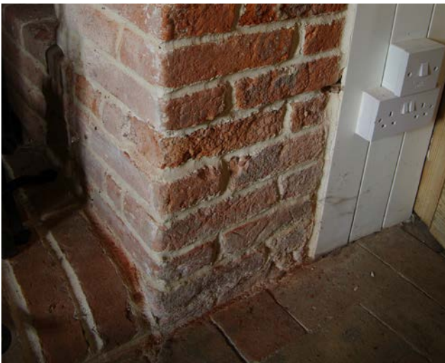
Figure 22: Spalling brickwork to inglenook fireplace due to aggressive cleaning.
