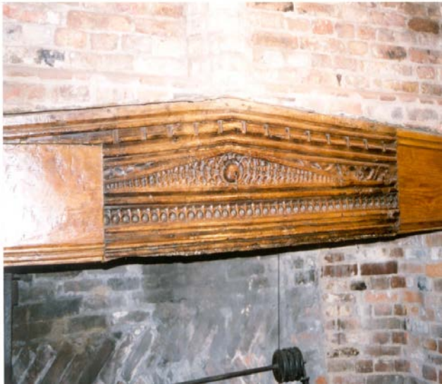
Figure 17: Repair is preferable to replacement, as with the repaired ends of this mantel beam. They respect the original but do not attempt to ape it. Photo: © Douglas D Kent
