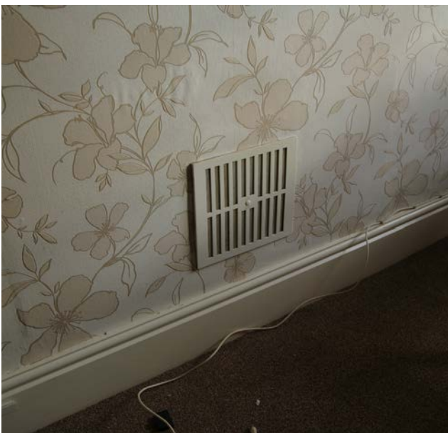
Figure 38: A redundant flue should be ventilated at the bottom where the fireplace opening is blocked off.
